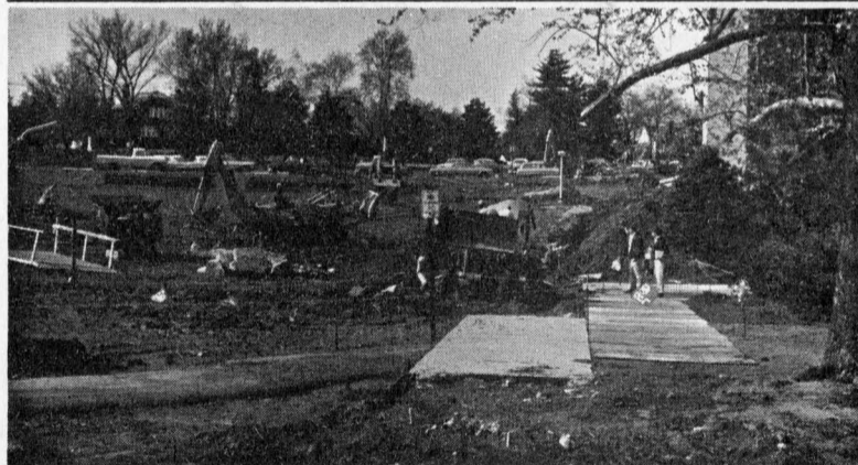
Work in the Benton Hall area, necessitating the removal of part of the sidewalk there, is part of the overall contract of the Mathematics-Languages Building and is designed to bring utilities, domestic water, a fire line, gas and telephone lines, to the new Mathematics-Languages Building and to the new Library. The utility link will be tested and ditches will be refilled by early summer.
